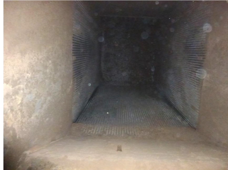
Furnace pass slagging after 12 weeks of operation with a Shock Pulse Generator (SPG)
