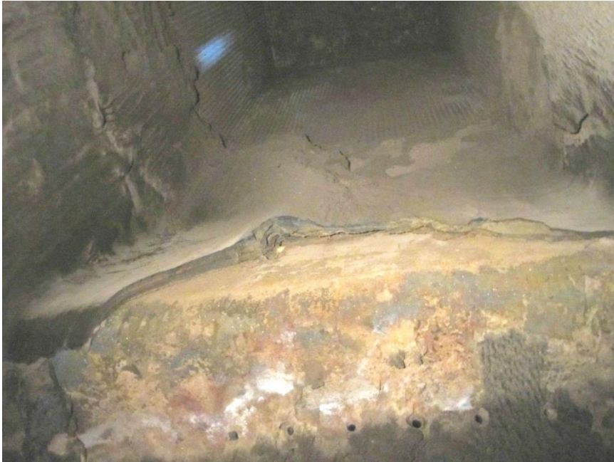
Furnace pass slagging after 10 weeks of operation
